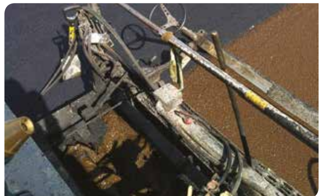
Fresh slurry is brown but cures to a black surface with an appearance similar to hot mix asphalt. Source: Duncor
