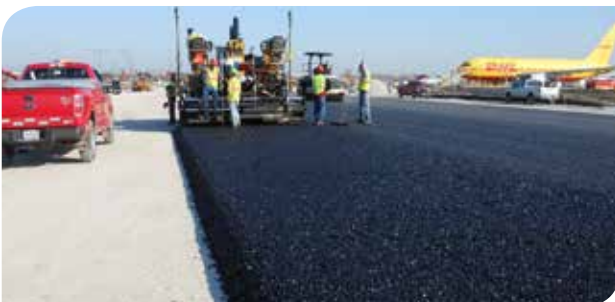
Use of Rediset LQ in a paving project at the Chicago O'Hare airport
