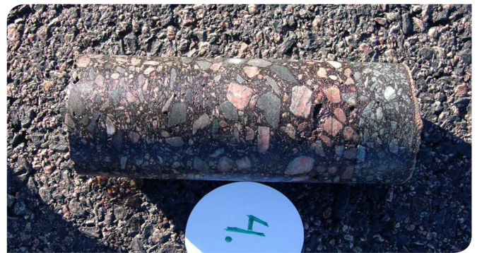
Core sample taken from the runway pavement used in the ITSM test
