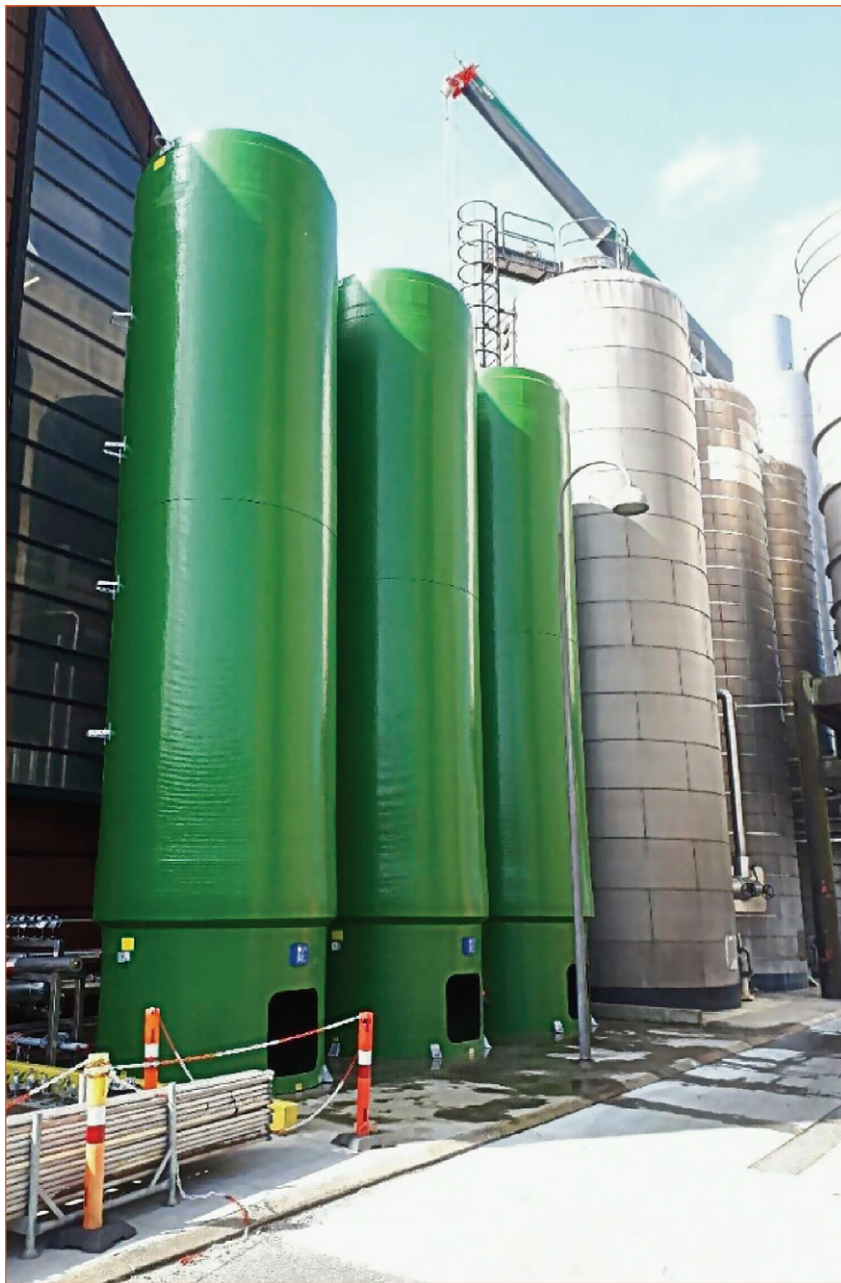
Fig. 1: The three storage tanks as installed
