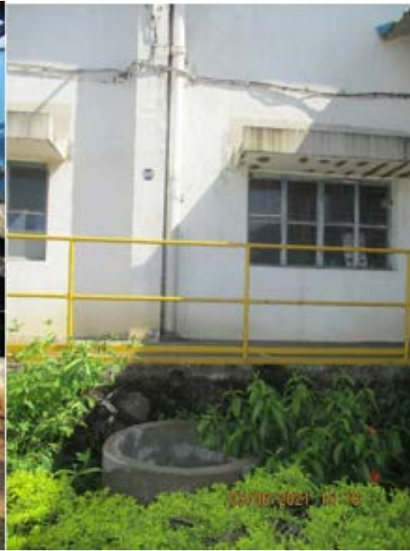
2. Rainwater recharge pit of Building roof
