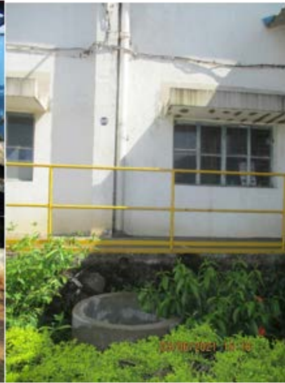
2. Rainwater recharge pit of Building roof
